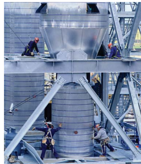
The company’s largest low-sulfur gasoline unit to date is at the Ferndale, Washington, refinery.
